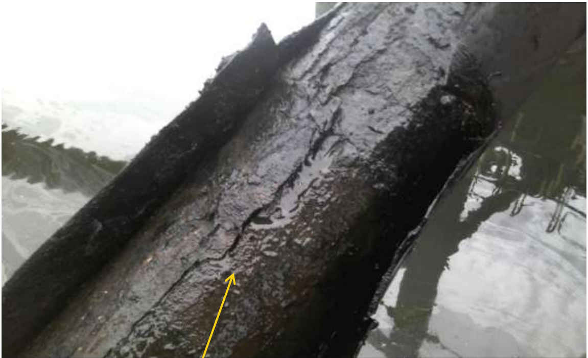
Overview: Part of spill impact on 6" Belema Pipeline right of way at Belema. Picture was taken during Joint Investigation of 25 th March 2014.
