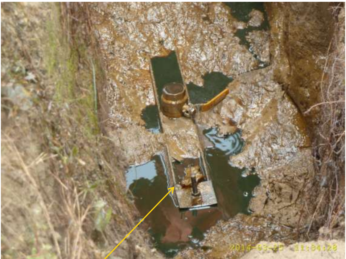
Close-up: Illegal fitting on 28" Nkpoku-Bomu Pipeline at Kpoghor. Picture was taken during Joint Investigation of 25 th March 2014.
