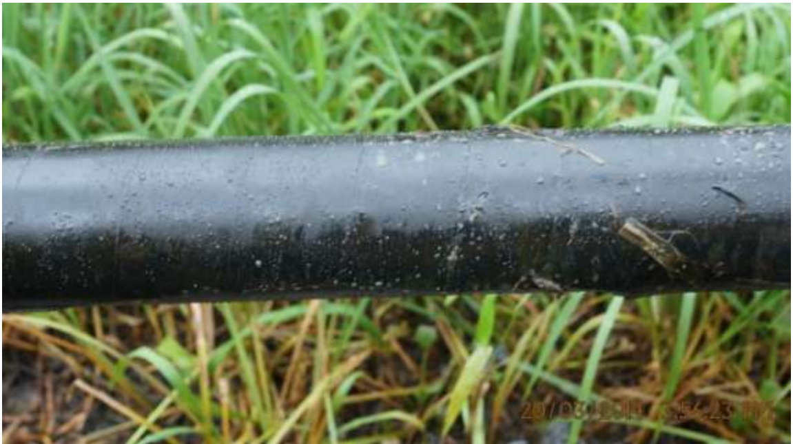
Close-up: Spill due to corrosion on Opukushi Well24T Flowline at Egbemo-Angalabiri. Picture was taken during Joint Investigation of 20 th March 2014.
