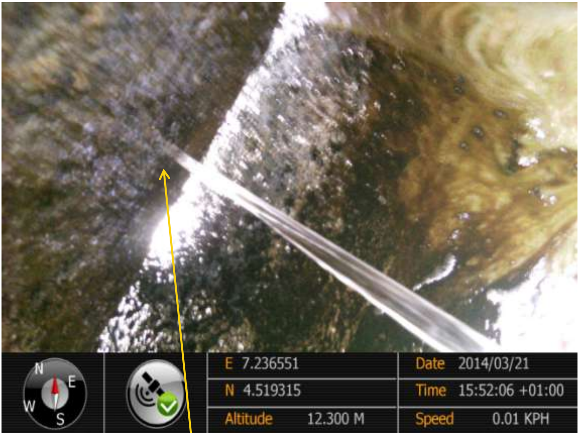
Close-up: Spill due to corrosion on 24" Bomu-Bonny Pipeline at Freetown. Picture was taken during Joint Investigation of 21 st March 2014.
