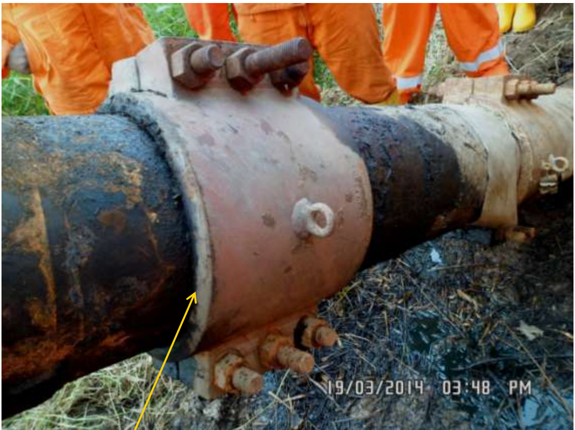
Close-up: Failed clamp on 10" Diebu Creek – Nun River Pipeline at Peremabiri. Picture was taken during Joint Investigation of 19 th March 2014.
