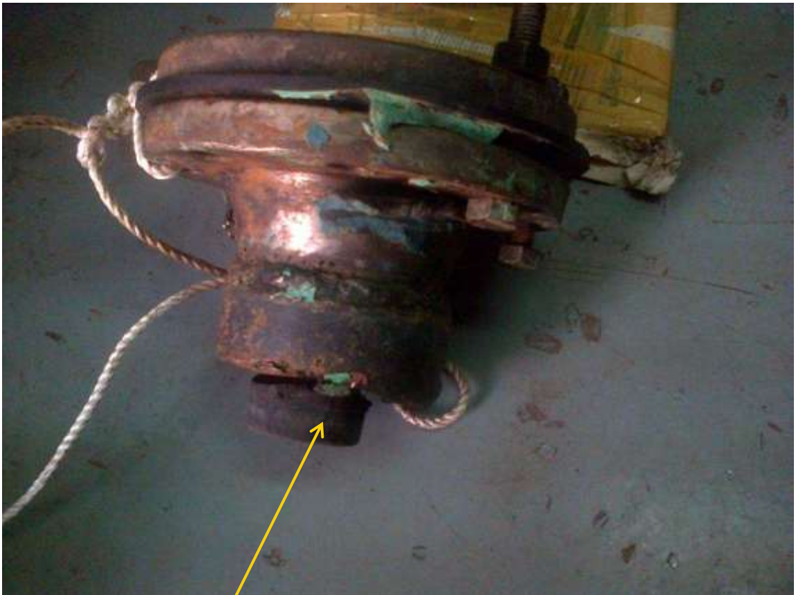
Close-up: Illegal fitting removed from underwater spill point on 48" Forcados Crude Oil Export Pipeline at Ogulagha.
