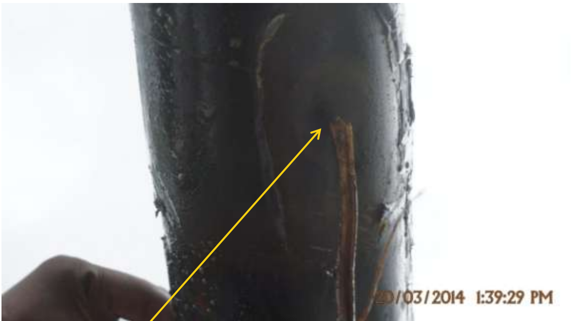
Close-up: Spill due to corrosion on Opukushi Well24T Flowline at Egbemo-Angalabiri. Picture was taken during Joint Investigation of 20 th March 2014.
