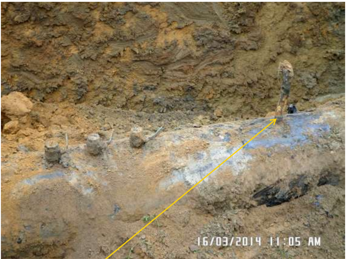
Close-up: Illegal fitting on 28" Nkpoku-Bomu Pipeline at Akpajo. Picture was taken during Joint Investigation of 16 th March 2014.
