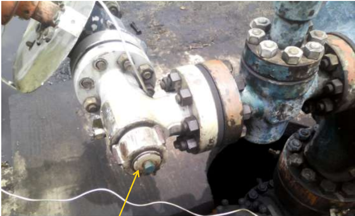
Overview: Part of spill impact on at ImoRiver2 Well28L Wellhead right of way at Umuedeokwara/Odagwa. Picture was taken during Joint Investigation of 6 th March 2014.
