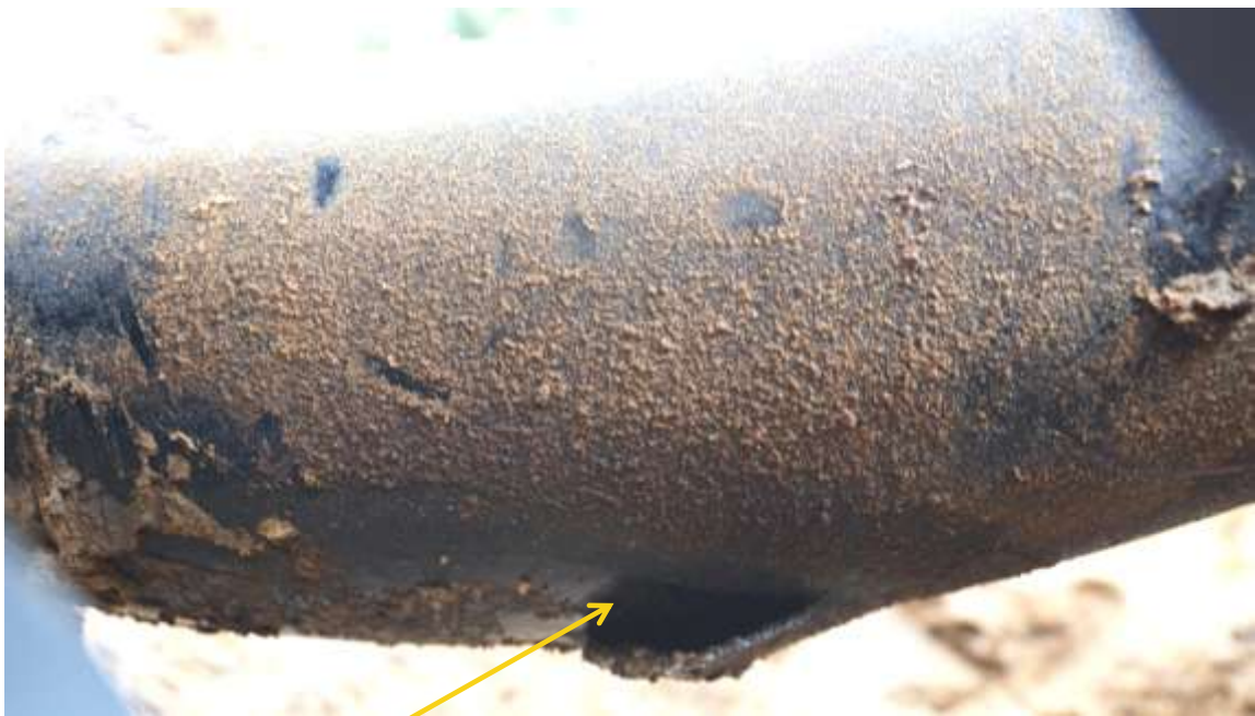
Close-up: Position of pinhole leak on Yokri Manifold8 LP2 Bulkhead at Yokri. Picture was taken during Joint Investigation of 7 th March 2014.
