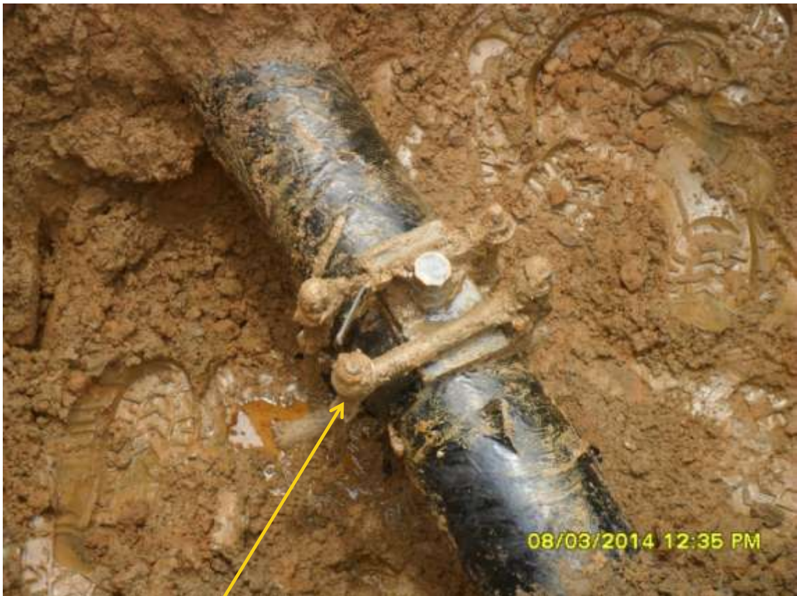
Close-up: Illegal fitting on 6" Obigbo North – Ogale Pipeline at Ogale. Picture was taken during Joint Investigation of 8 th March 2014.
