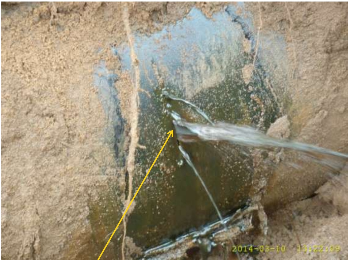
Close-up: Hacksaw cut on 24" Nkpoku-Bomu Trans Niger Pipeline at Biara. Picture was taken during Joint Investigation of 10th March 2014.
