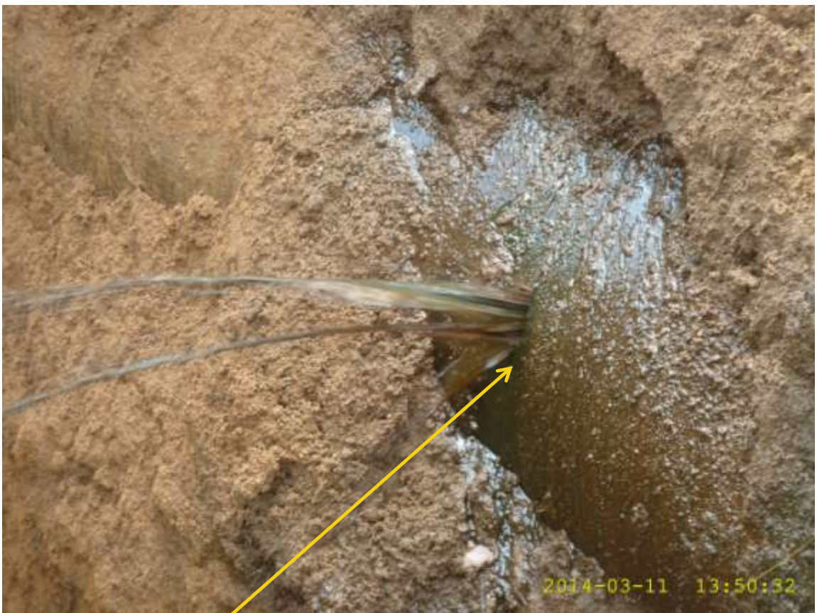
Close-up: Hacksaw cut on 24" Nkpoku-Bomu Trans Niger Pipeline at Biara. Picture was taken during Joint Investigation of 11 th March 2014.
