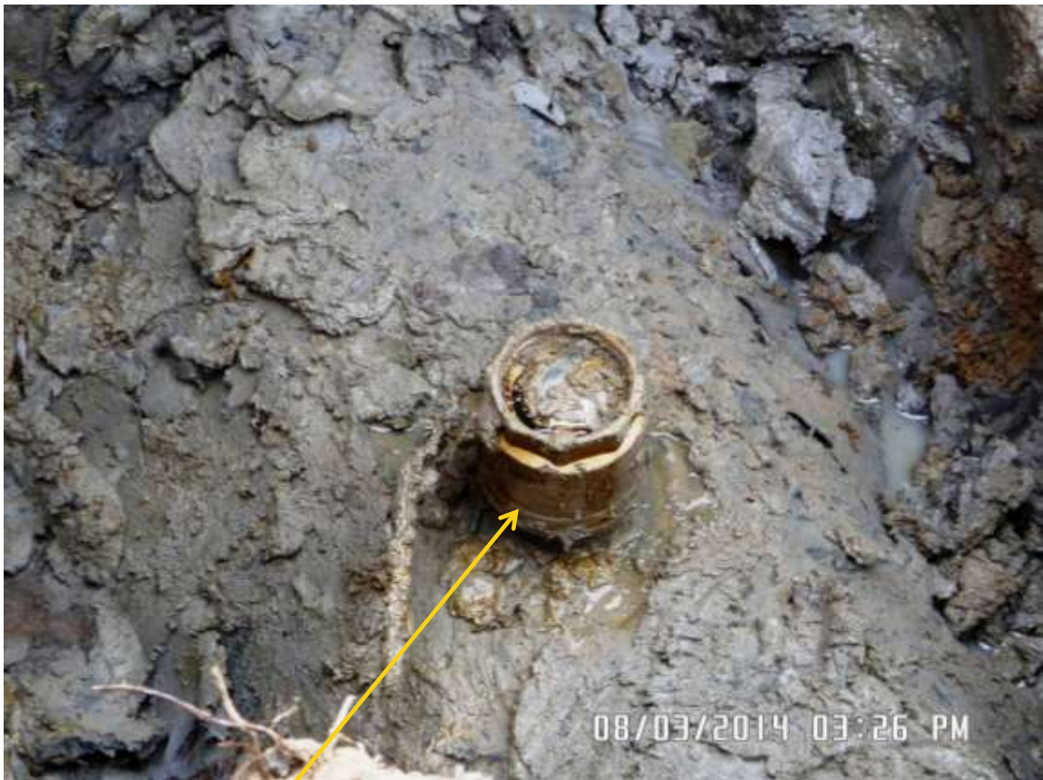
Close-up: Illegal fitting on 24" Bomu-Bonny Pipeline at Bodowest. Picture was taken during Joint Investigation of 8th March 2014.
