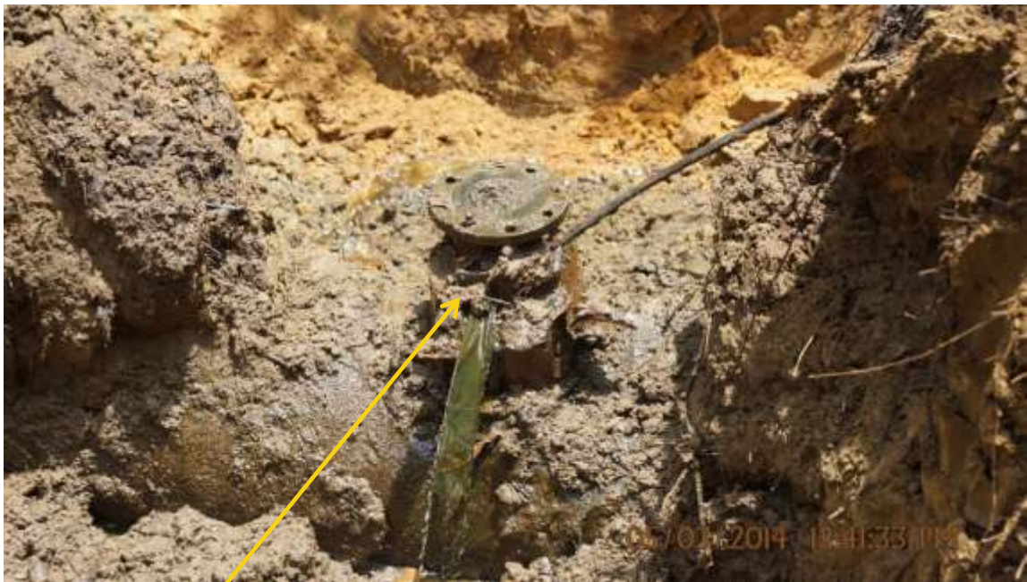
Close-up: Illegal fitting on 20" Otumara-Escravos Pipeline at Adjudaibo. Picture was taken during Joint Investigation of 5th March 2014.
