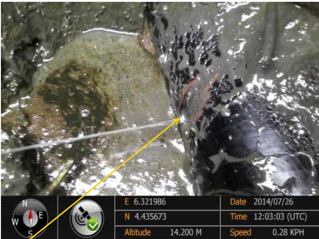
Close-up: Spill due to corrosion on Nembe 1 Well 23T Flowline at Nembe Creek . Picture was taken during Joint Investigation of 26 th July 2014.
