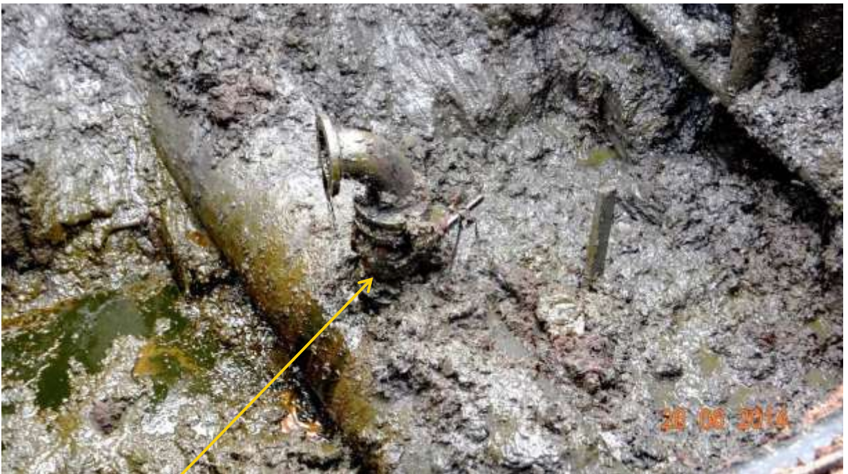
Close-up: Illegal fitting on 24" Cawthorne – Channel – Bonny Pipeline at Adamakiri. Picture was taken during Joint Investigation of 26 th June 2014
