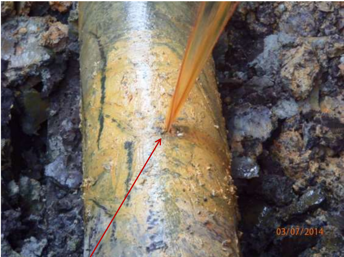
Close-up: Spill Point1 on 10" Diebu Creek – Nun River Pipeline at Onyoma/Enewari. Picture was taken during Joint Investigation of 3 rd July 2014
