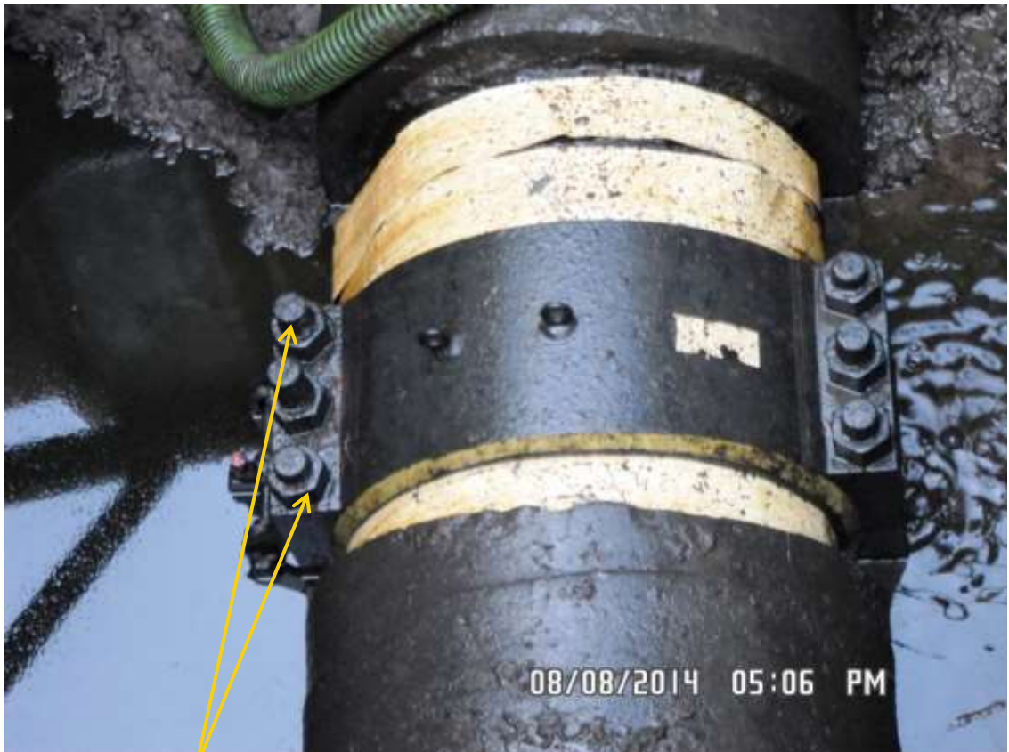
Close-up: Loosened bolts on 30" Nembe Creek Pipeline at Boro. Picture was taken during Joint Investigation of 8 th August 2014.
