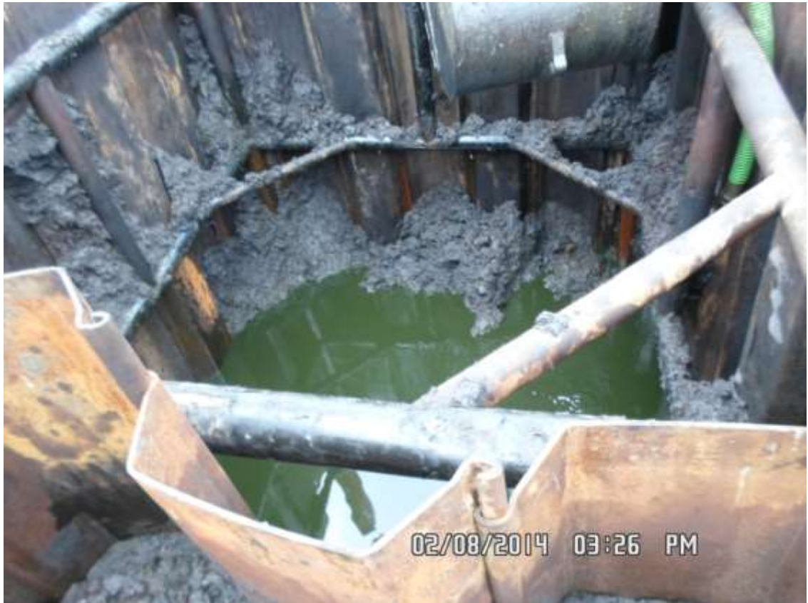
Overview: Part of spill impact on 30" Nembe Creek Pipeline Right of Way at Boro. Picture was taken during Joint Investigation of 2 nd August 2014.
