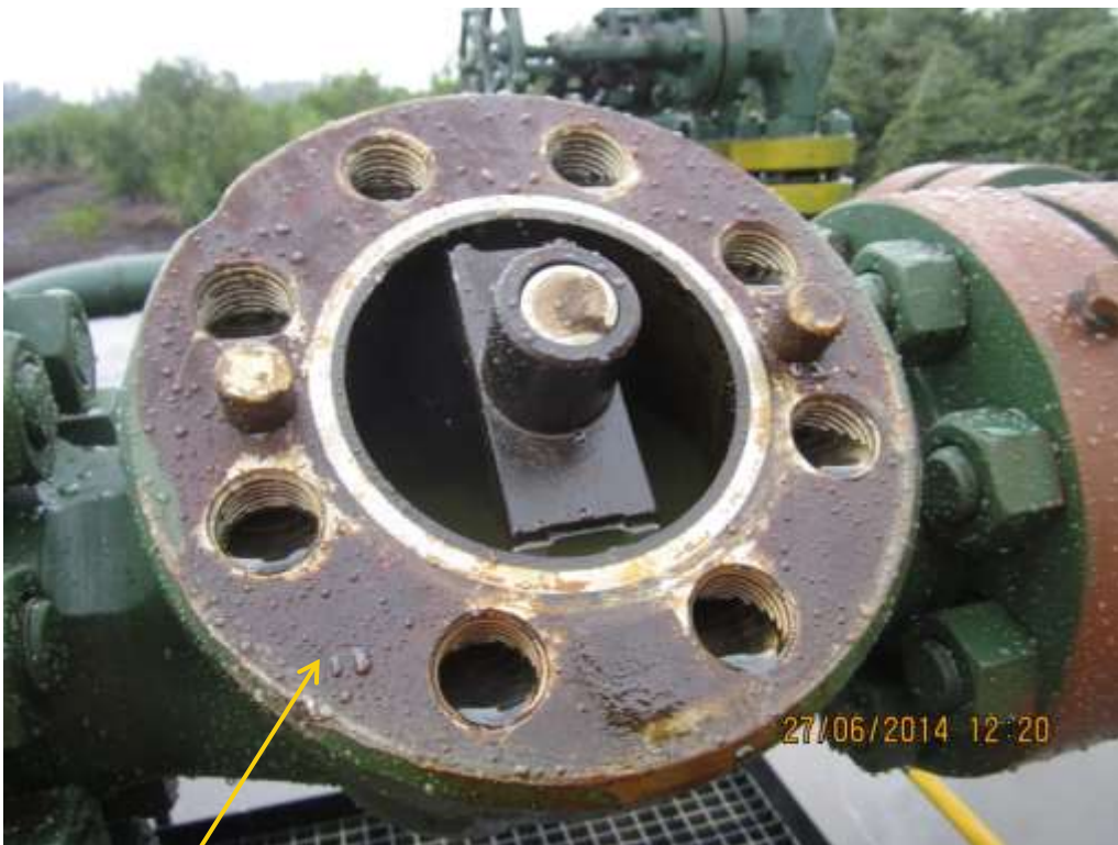
Close-up: Former position of Control unit removed from Belema Well9T Wellhead at Belema. Picture was taken during Joint Investigation of 27 th June 2014
