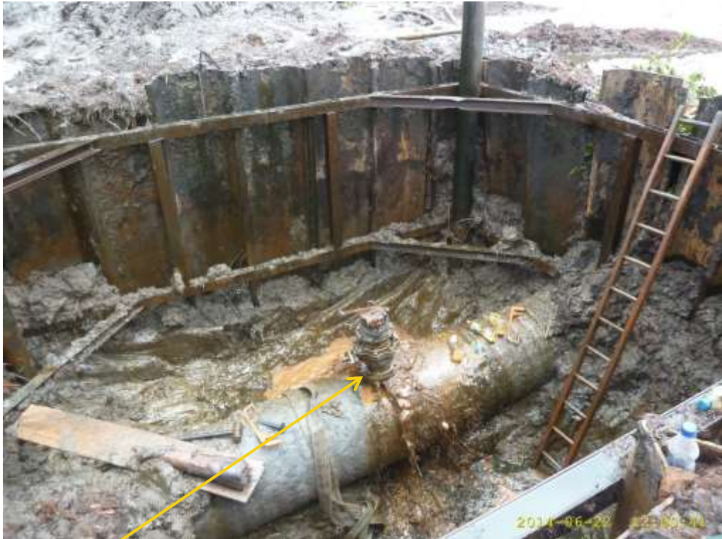
Close-up: Illegal fitting on 28" Bomu-Bonny Trans Niger Pipeline at Owokiri. Picture was taken during Joint Investigation of 22 nd June 2014.
