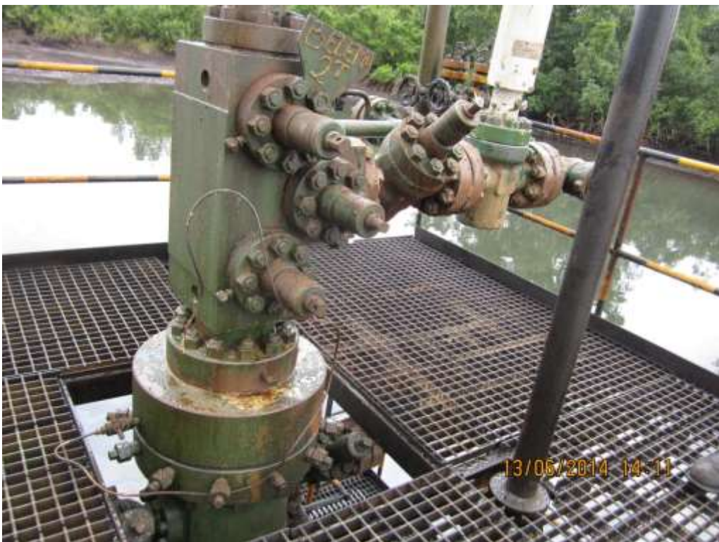
Close-up: Control unit missing from Belema Well2T Wellhead at Belema. Picture was taken during Joint Investigation of 13 th June 2014.
