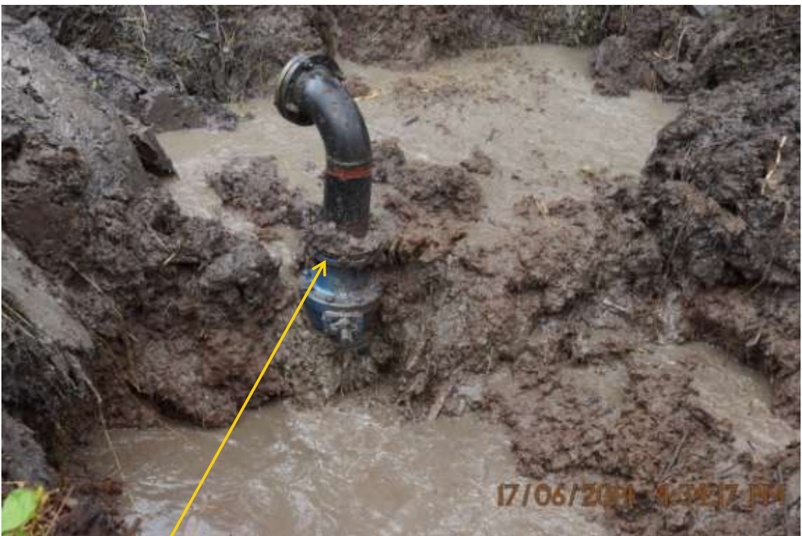
Close-up: Illegal fitting on 20" Opukushi-Brass Creek Pipeline at Tamogbene. Picture was taken during Joint Investigation of 17 th June 2014.
