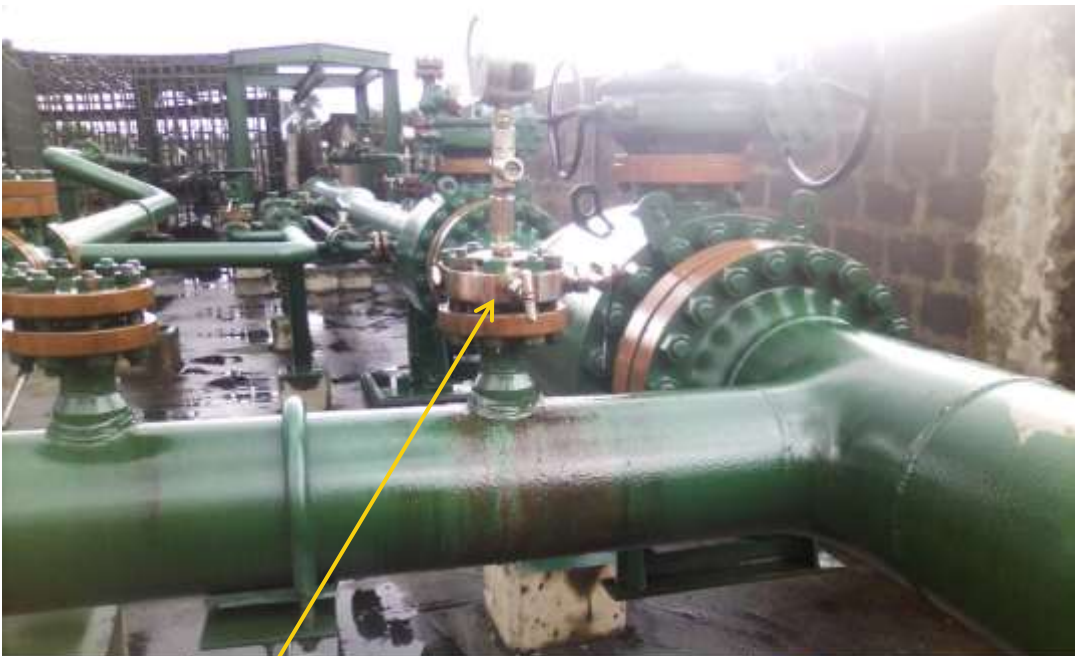
Overview: Part of spill impact on 12" Adibawa-Okordia Manifold Right of Way at Ikarama/Okordia. Picture was taken during Joint Investigation of 13 th June 2014.
