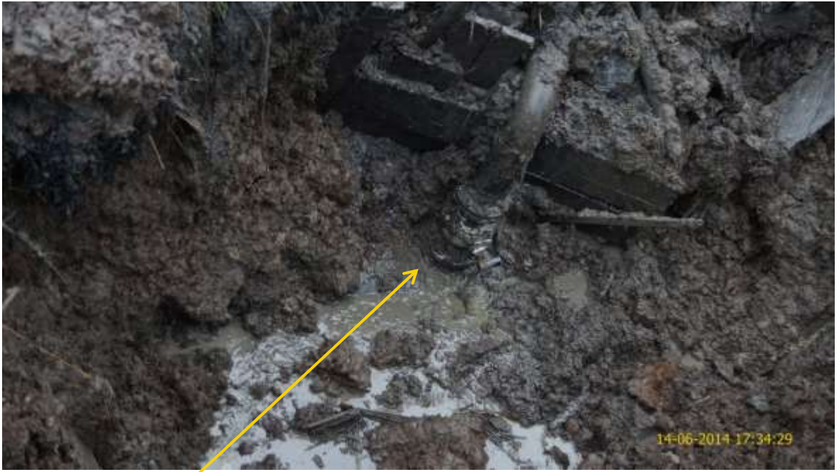
Close-up: Illegal fitting on 20" Opukushi – Brass Creek Pipeline at Tamogbene. Picture was taken during Joint Investigation of 14 th June 2014.
