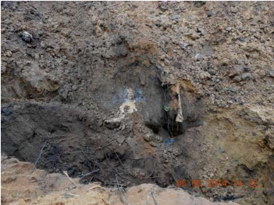
Overview: Spill clearly visible after excavation on 36" Nkpoku-Bomu Pipeline at Atali. Picture was taken during Joint Investigation of 6 th June 2014.
