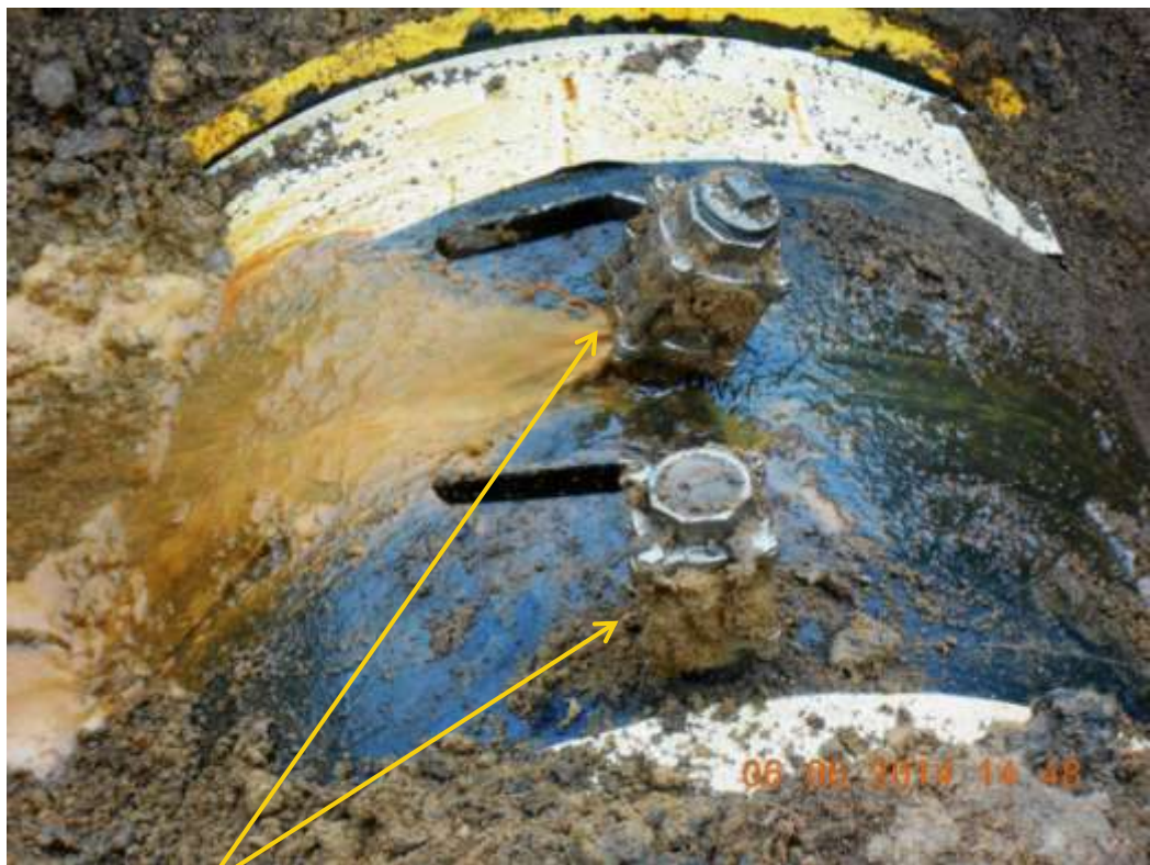
Close-up: Illegal fittings on 36" Nkpoku-Bomu Pipeline at Atali. Picture was taken during Joint Investigation of 6 th June 2014.
