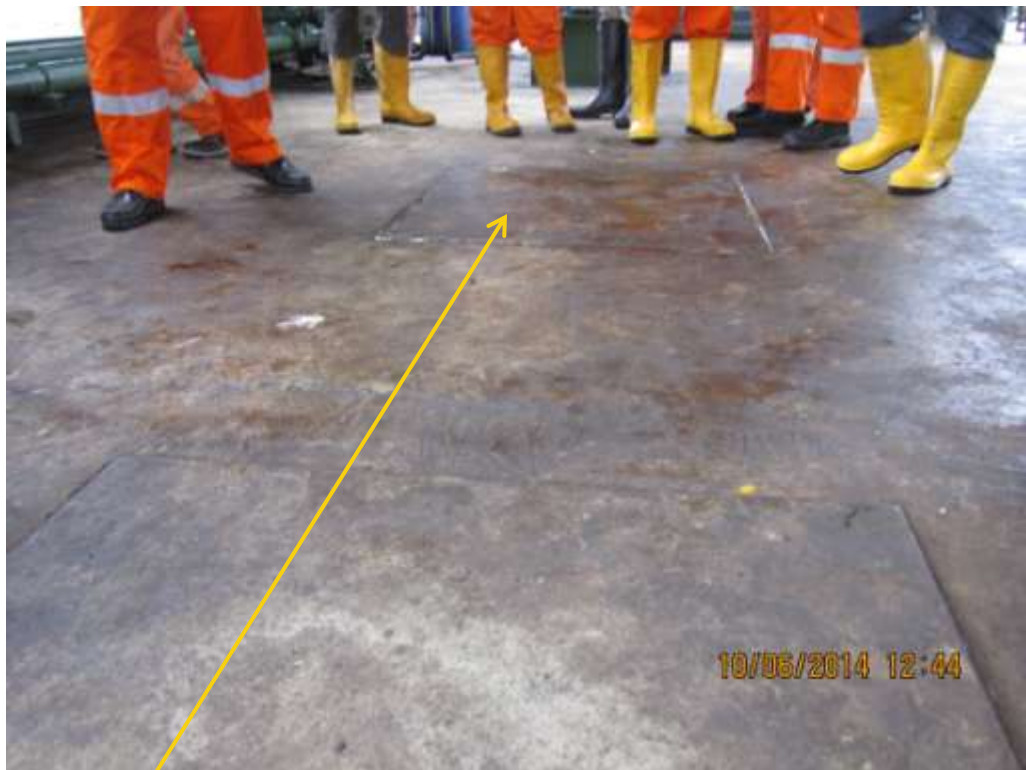
Close-up: Cover of closed drain at Santa Barbara Mobile Production Facility. Picture was taken during Joint Investigation of 10 th June 2014.
