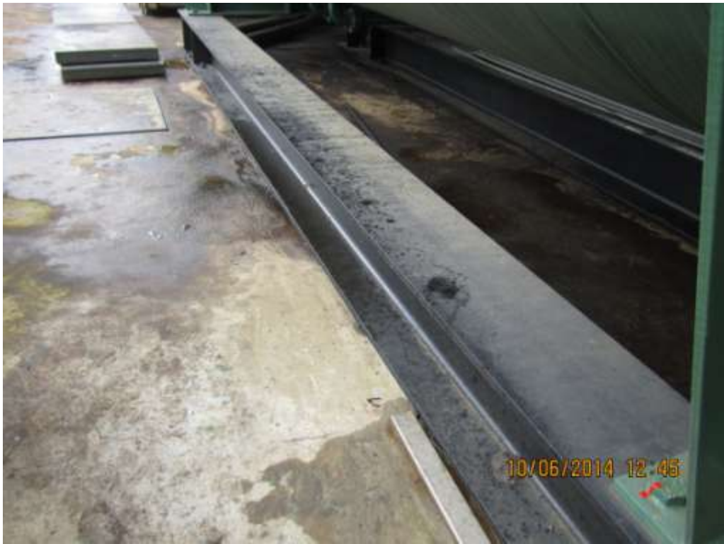
Overview: Oil stains on concrete surface at Santa Barbara Mobile Production Facility. Picture was taken during Joint Investigation of 10 th June 2014.
