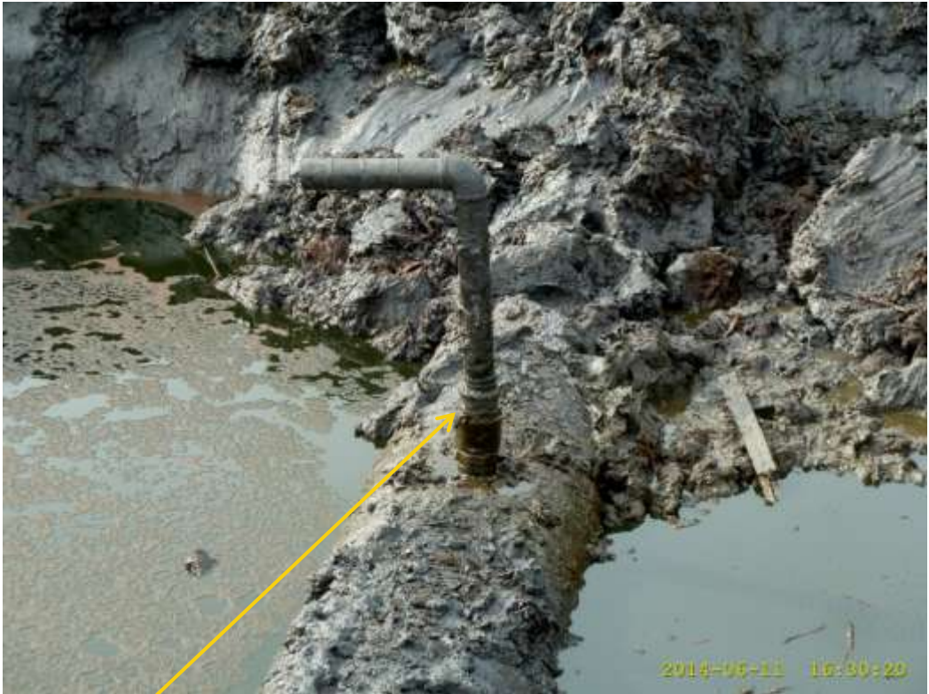
Close-up: Illegal fitting on 28" Bomu-Bonny Trans Niger Pipeline. Picture was taken during Joint Investigation of 11 th June 2014.
