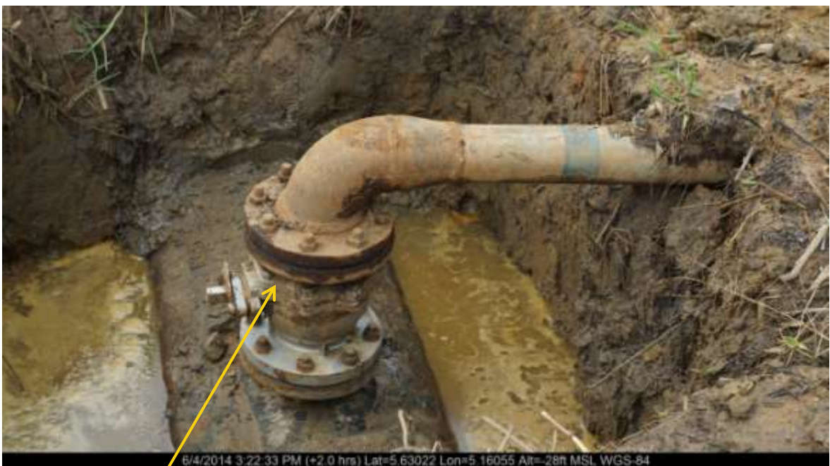
Close-up: Illegal fitting on 20" Otumara – Escravos Pipeline ta Ugboegungun. Picture was taken during Joint Investigation of 4 th June 2014.
