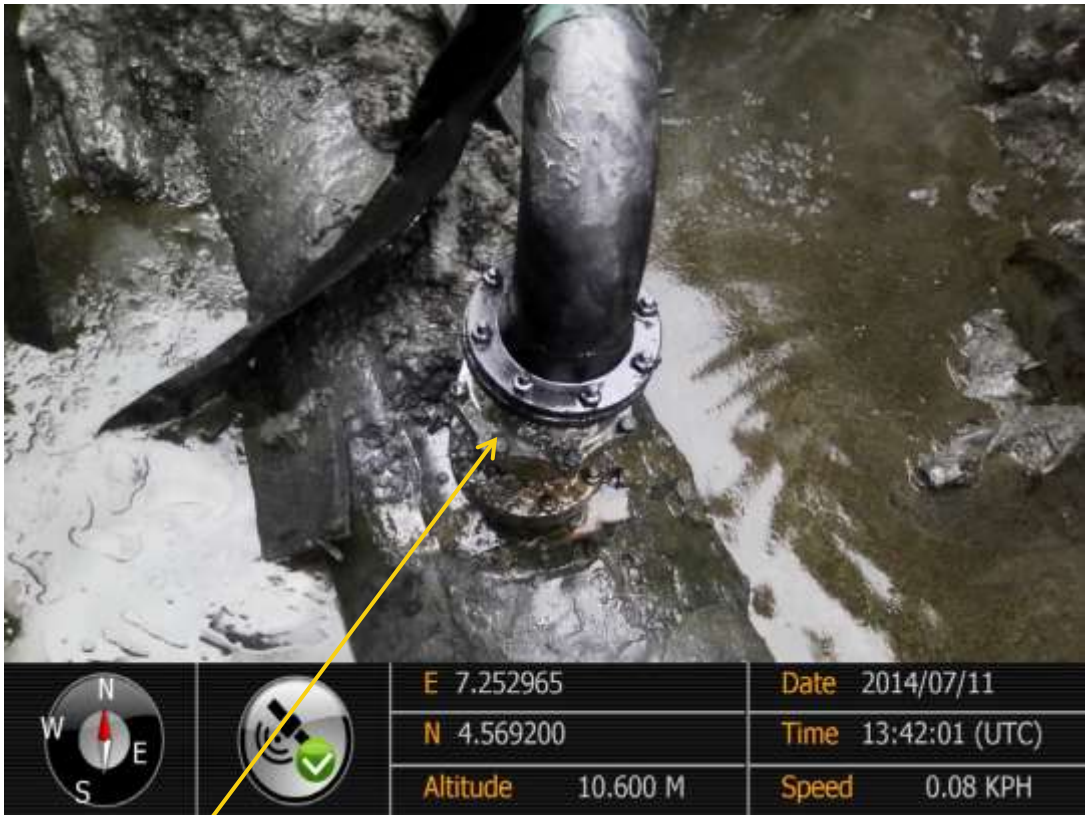
Close-up: Illegal fitting on 28" Bomu-Bonny Pipeline at Owokiri. Picture was taken during Joint Investigation of 11 th July 2014
