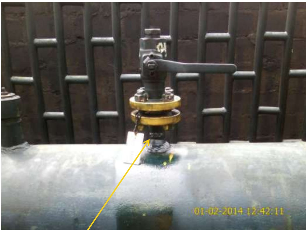
Close-up: Tampered valve on Okordia Manifold at Ikarama/Okordia. Picture was taken during Joint Investigation of 1st February 2014.
