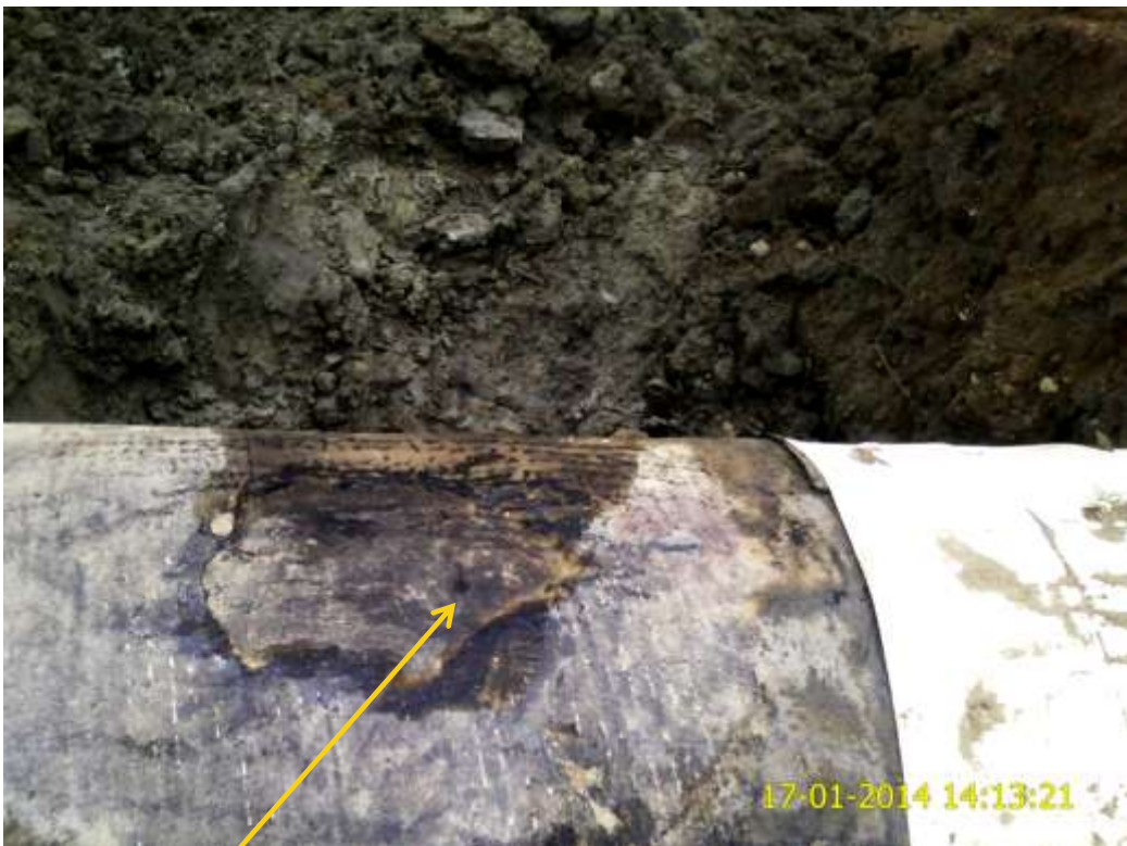
Close-up: Drilled hole on 24" Nkpoku-Bomu Pipeline at B-Dere. Picture was taken during Joint Investigation of 17 th January 2014.
