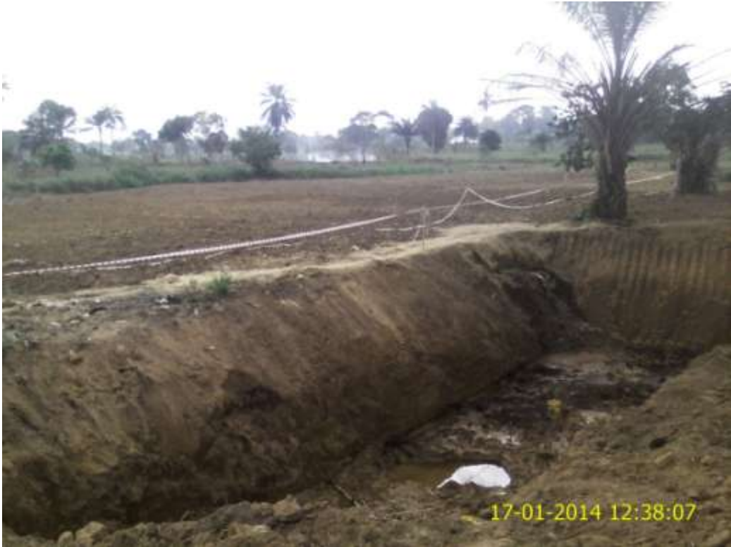
Overview: Part of spill impact on 24" Nkpoku-Bomu Pipeline right of way at B-Dere. Picture was taken during Joint Investigation of 17 th January 2014.
