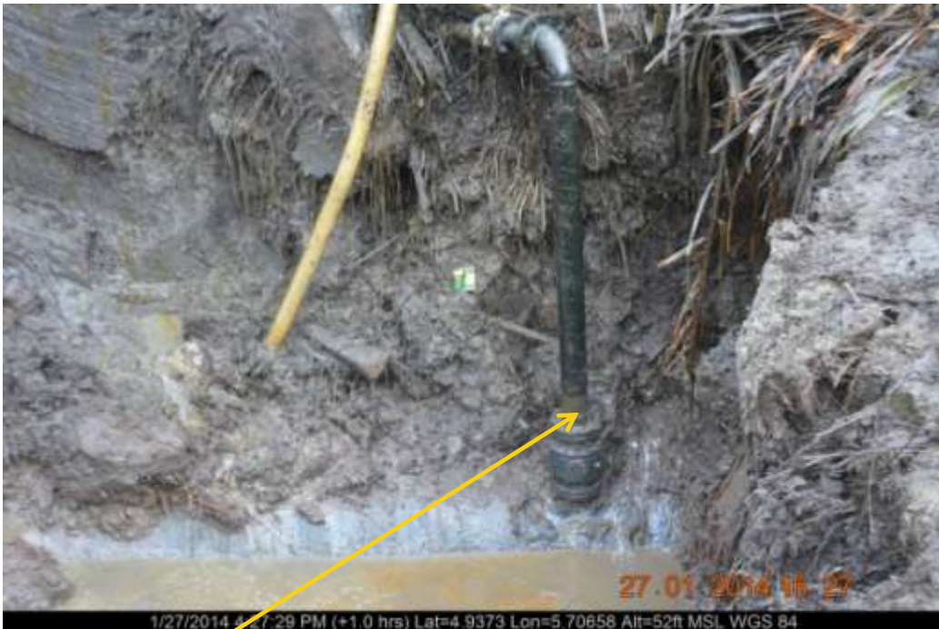
Close-up: Illegal fitting on 20" Opukushi – Brass Creek Pipeline at Tamogbene. Picture was taken during Joint Investigation of 27 th January 2014.
