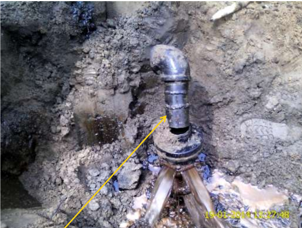
Close-up: Illegal fitting on 28" Nkpoku-Bomu Pipeline at Kporghor. Picture was taken during Joint Investigation of 19th January 2014.
