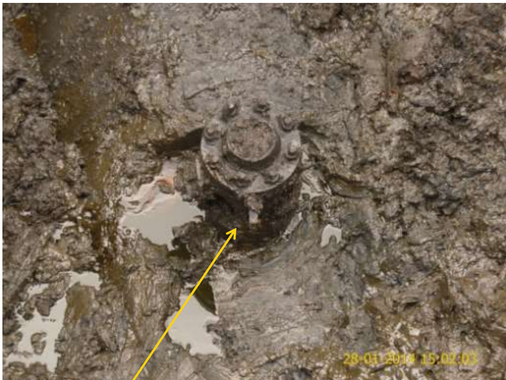
Close-up: Illegal fitting on 30" Nembe Creek Pipeline at Elem-Kalabari. Picture was taken during Joint Investigation of 28 th January 2014.
