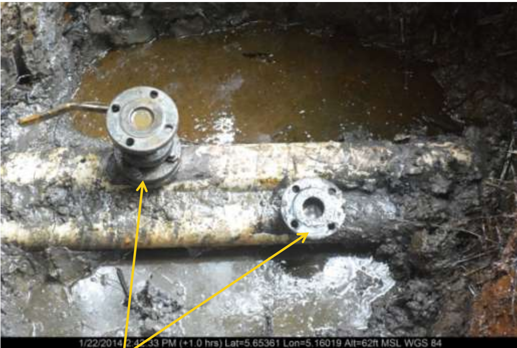
Close-up: Illegal fittings on Otumara Well34L/S Flowline at Ugboegungun. Picture was taken during Joint Investigation of 22nd January 2014.
