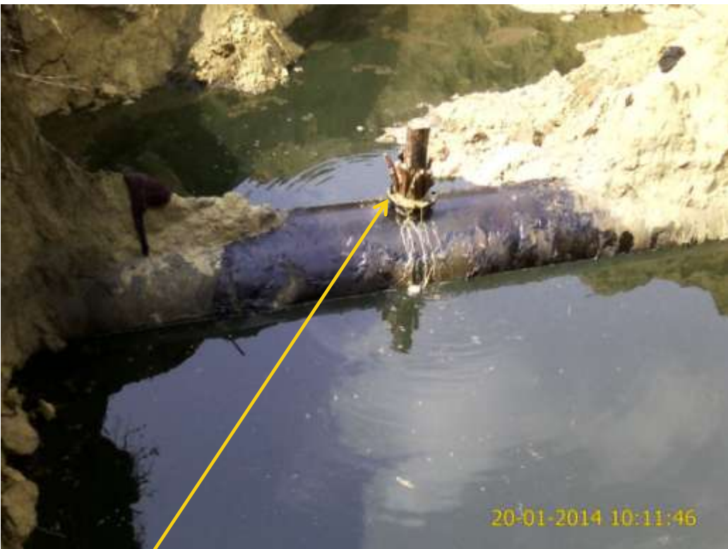
Close-up: Illegal fitting on 28" Nkpoku-Bomu Pipeline at Ekporo. Picture was taken during Joint Investigation of 20th January 2014.
