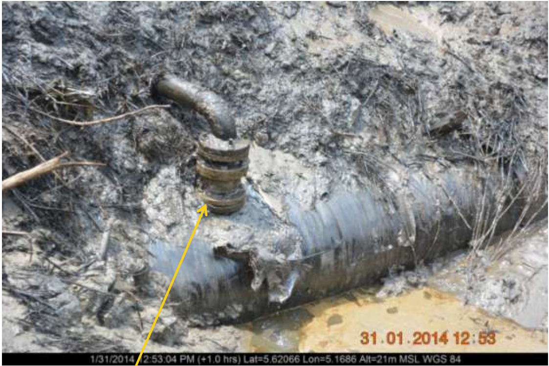
Close-up: Leaking illegal fitting on 20" Otumara-Escravos Pipeline at Ugboegungun. Picture was taken during Joint Investigation of 31 st January 2014.
