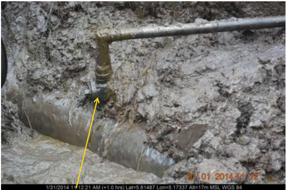
Close-up: Non-leaking illegal fitting on 20" Otumara-Escravos Pipeline at Ugboegun. Picture was taken during Joint Investigation of 31 st January 2014.
