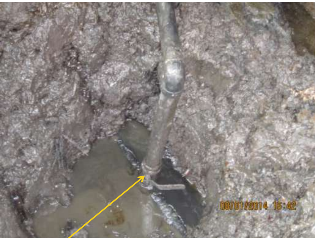
Close-up: Illegal fitting on Santa Barbara Well6T Flowline at Ikegimakiri. Picture was taken during Joint Investigation of 8th January 2014.
