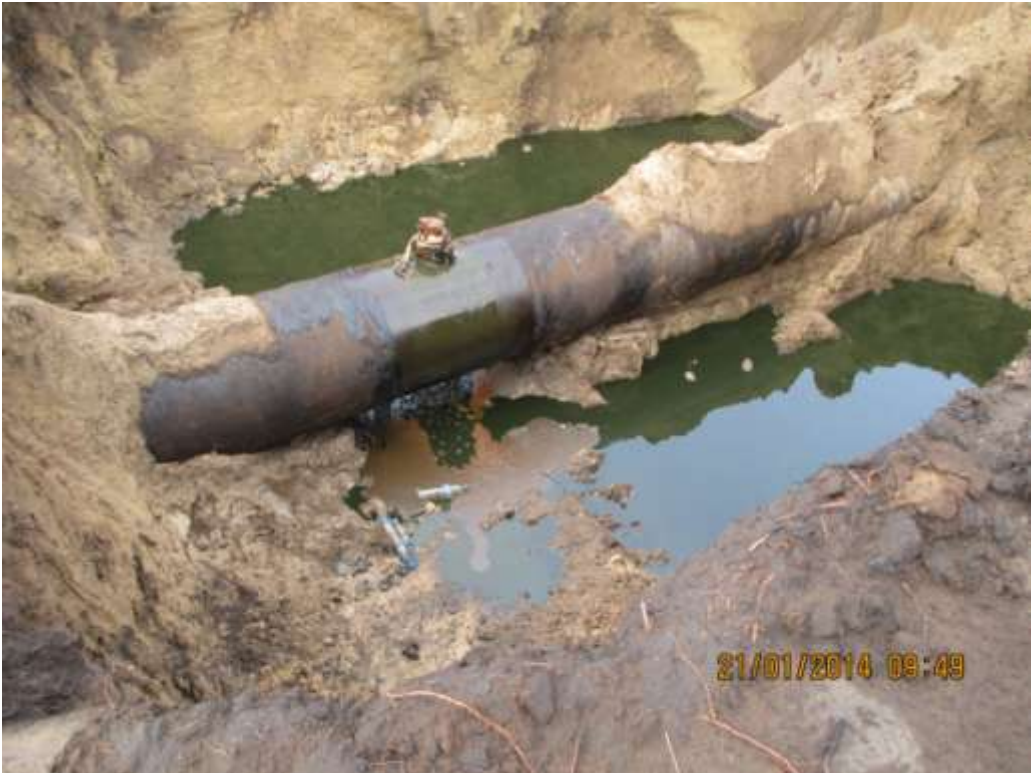
Overview: Part of spill impact on 28" Nkpoku-Bomu Pipeline right of way at Ekporo. Picture was taken during Joint Investigation of 21 st January 2014.
