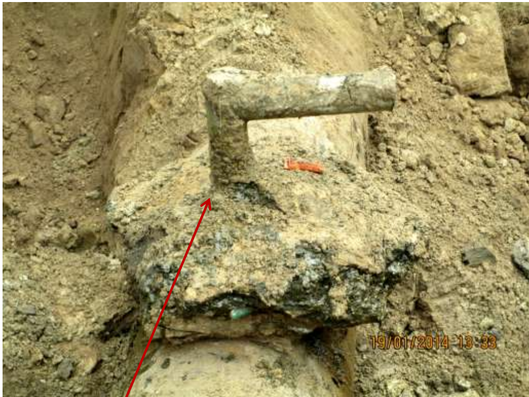
Closeup: Illegal fitting on 28" Nkpoku-Bomu Pipeline right of way at Ekporo. Picture was taken during Joint Investigation of 19th January 2014.
