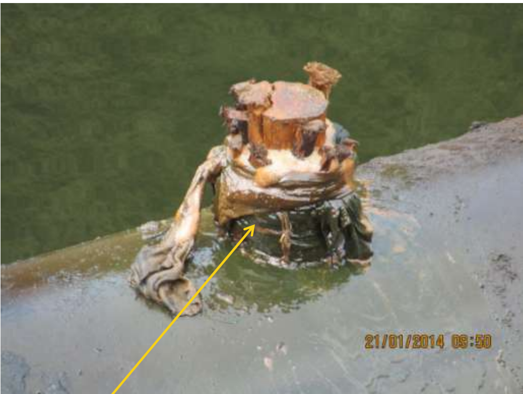
Close-up: Illegal fitting on 28" Nkpoku-Bomu Pipeline at Ekporo. Picture was taken during Joint Investigation of 21 st January 2014.
