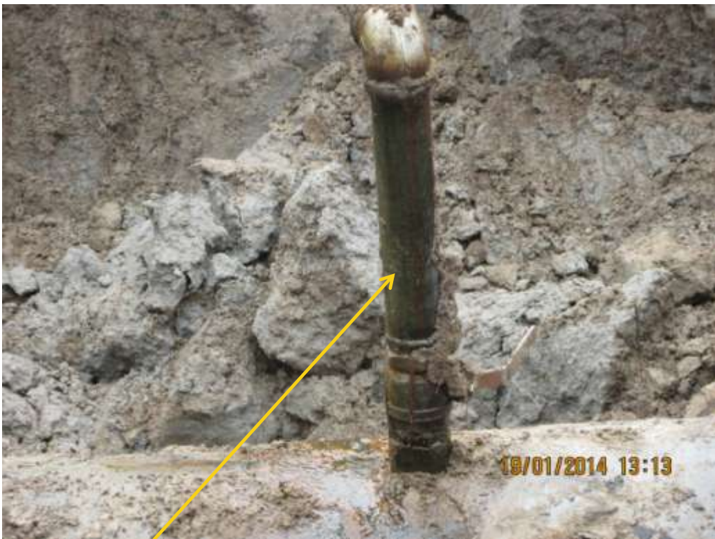
Close-up: Illegal fitting on 28" Nkpoku-Bomu Pipeline at Ekporo. Picture was taken during Joint Investigation of 19th January 2014.
