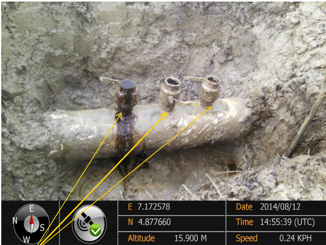
Close-up: Illegal fittings on 12" Imo River – Ogale Pipeline at Komkom . Picture was taken during Joint Investigation of 12 th August 2014.
