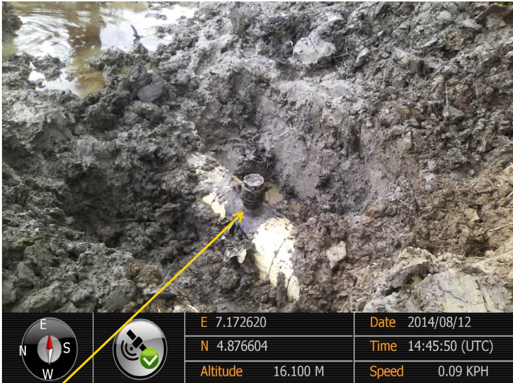
Close-up: Illegal fitting on 12" Imo River – Ogale Pipeline at Komkom . Picture was taken during Joint Investigation of 12 th August 2014.
