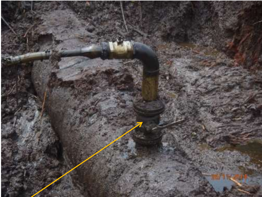
Close-up: Illegal fitting (spill point) on 28" Bomu-Bonny Pipeline at Oloma. Picture was taken during Joint Investigation of 26 th November 2014.
