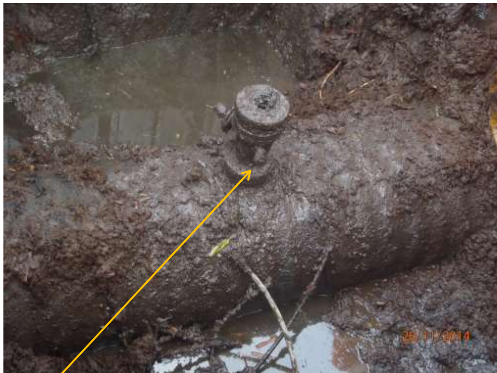
Close-up: Illegal fitting (non-leaking) on 28" Bomu-Bonny Pipeline at Oloma. Picture was taken during Joint Investigation of 26 th November 2014.
