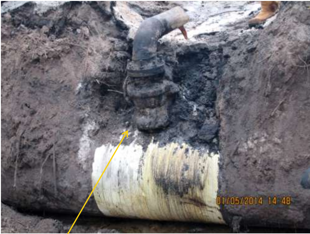
Close-up: Illegal fitting on 28" Nkpoku-Bomu Pipeline at B-Dere. Picture was taken during Joint Investigation of 1 st May 2014.
