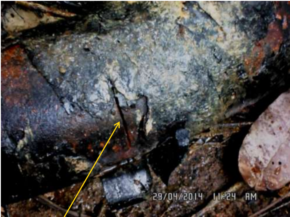
Close-up: Hacksaw cut on 4" Nun River Well10T Flowline at Oporoma. Picture was taken during Joint Investigation of 29 th April 2014.
