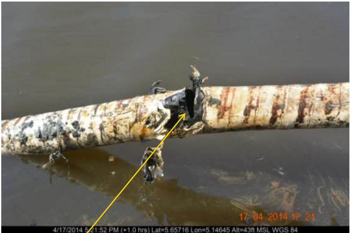
Close-up: Tear on Otumara Well41S Flowline at Ugboegungun. Picture was taken during Joint Investigation of 17 th April 2014.
