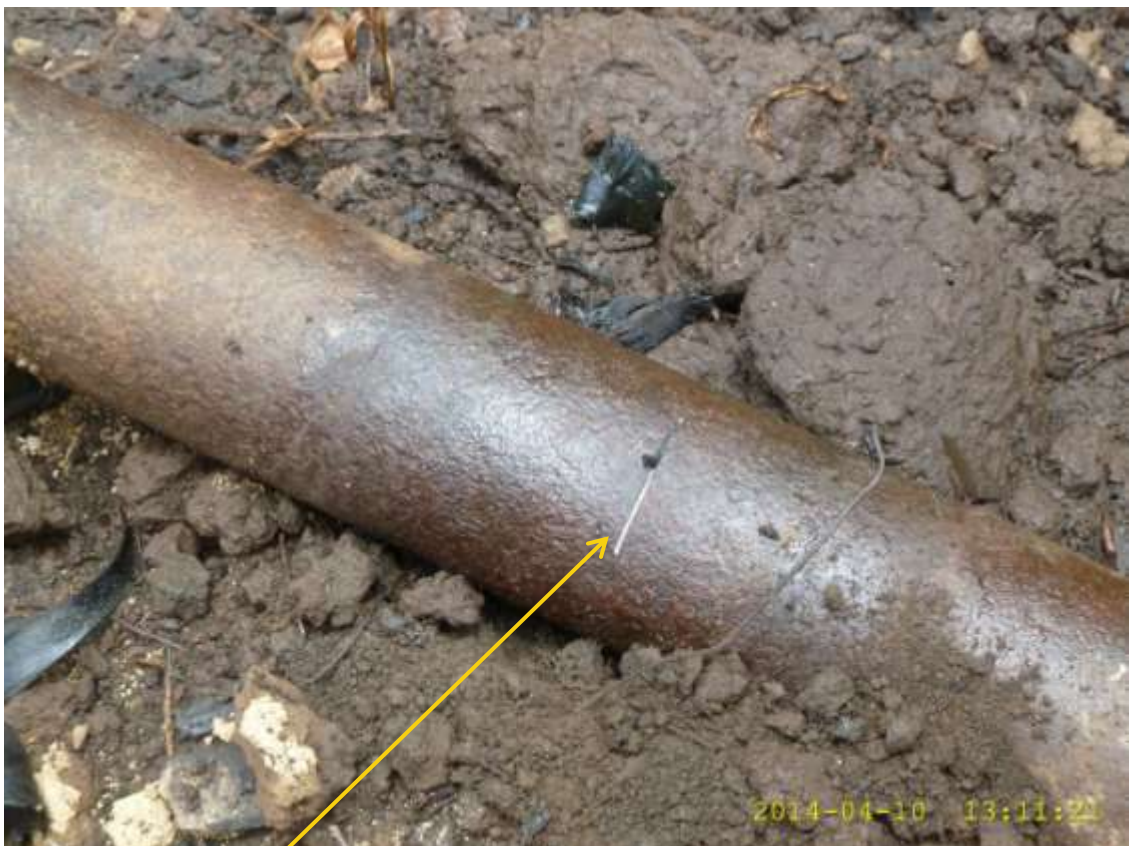
Close-up: Hacksaw cut on 4" Adibawa Well10S Flowline at Adibawa. Picture was taken during Joint Investigation of 10 th April 2014.
