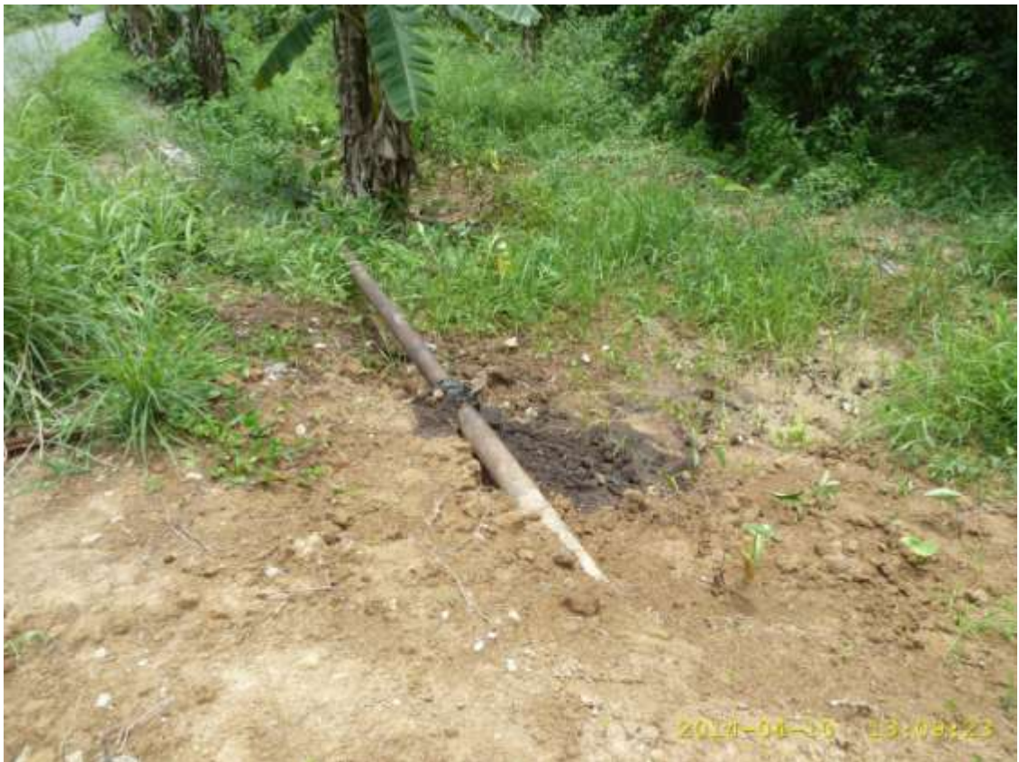
Overview: Part of spill impact on 4" Adibawa Well10S Flowline right of way at Adibawa. Picture was taken during Joint Investigation of 10 th April 2014.
