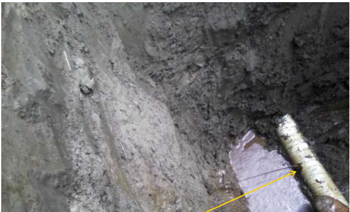
Overview: Part of spill impact on 4" Obele-Ibaa Pipeline right of way at Omueze/Ibaa. Picture was taken during Joint Investigation of 8 th April 2014.
