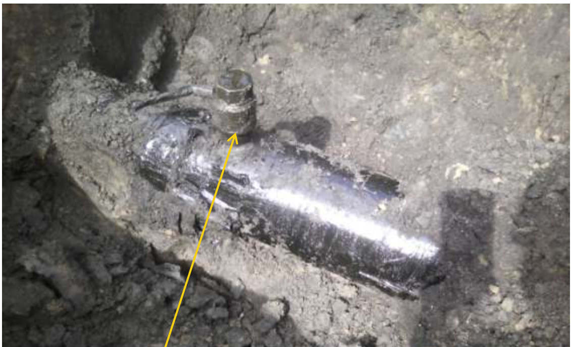
Overview: Part of spill impact on 8" Obigbo North – KomKom Pipeline right of way at Oyigbo. Picture was taken during Joint Investigation of 5 th April 2014.
