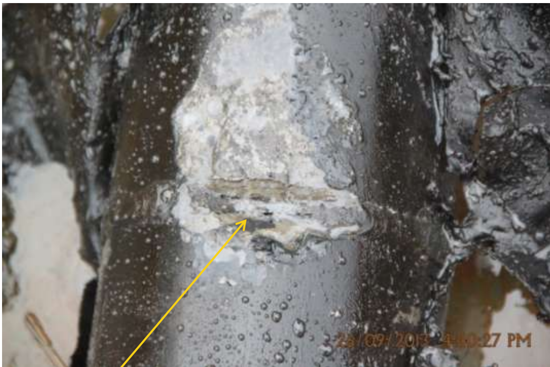
Close up: External corrosion on Kanbo Well7S flowline at Egbemoangarabiri/Agbidiama. Picture was taken during Joint Investigation of 26 th September 2013.
